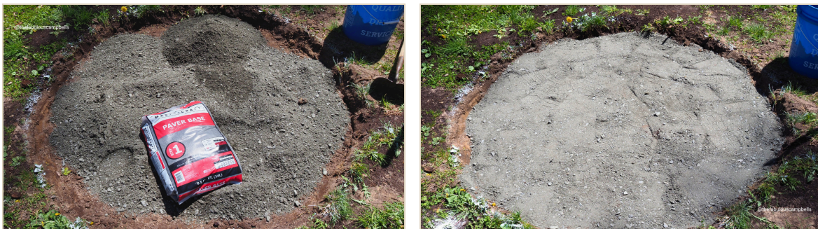
Emptying the first layer of paver base over the packed earth and tamping it perfectly flat.
